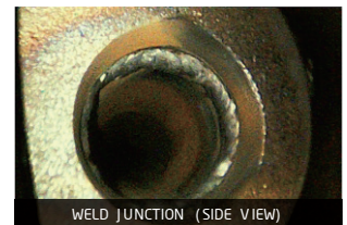
WELD JUNCTION (SIDE VIEW)
